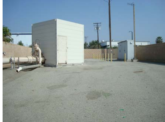
Existing Well No. 19 is located in the City of Chino Hills, north of Anderson Street. The well pump/motor is located behind the acoustical paneling.
