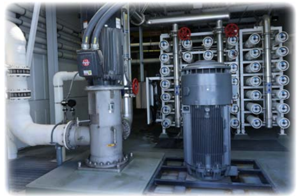
Filtration System at the Chino Desalter Authority I Facility
