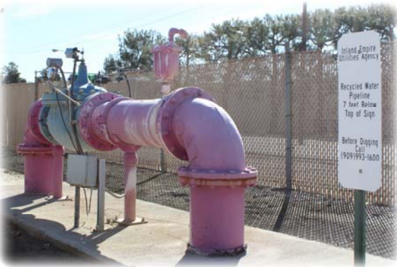
Recycled water line at the Ely Basins.
