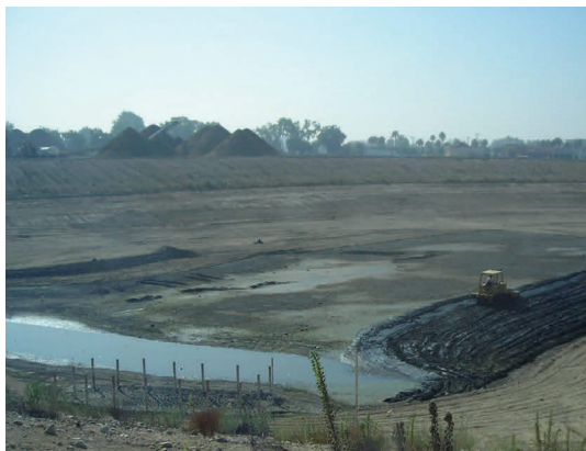
Turner Basins Recharge Expansion Project Excavation Milliken Grade Separation Stockpiles in Background
