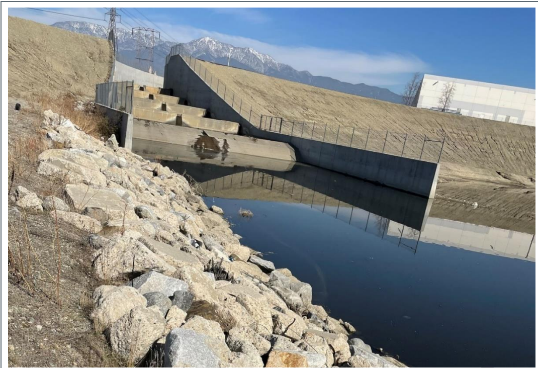
Photo 3 Rock Slope Protection on Conservation Berm East (Water) Side Slope at Inflow Structure
