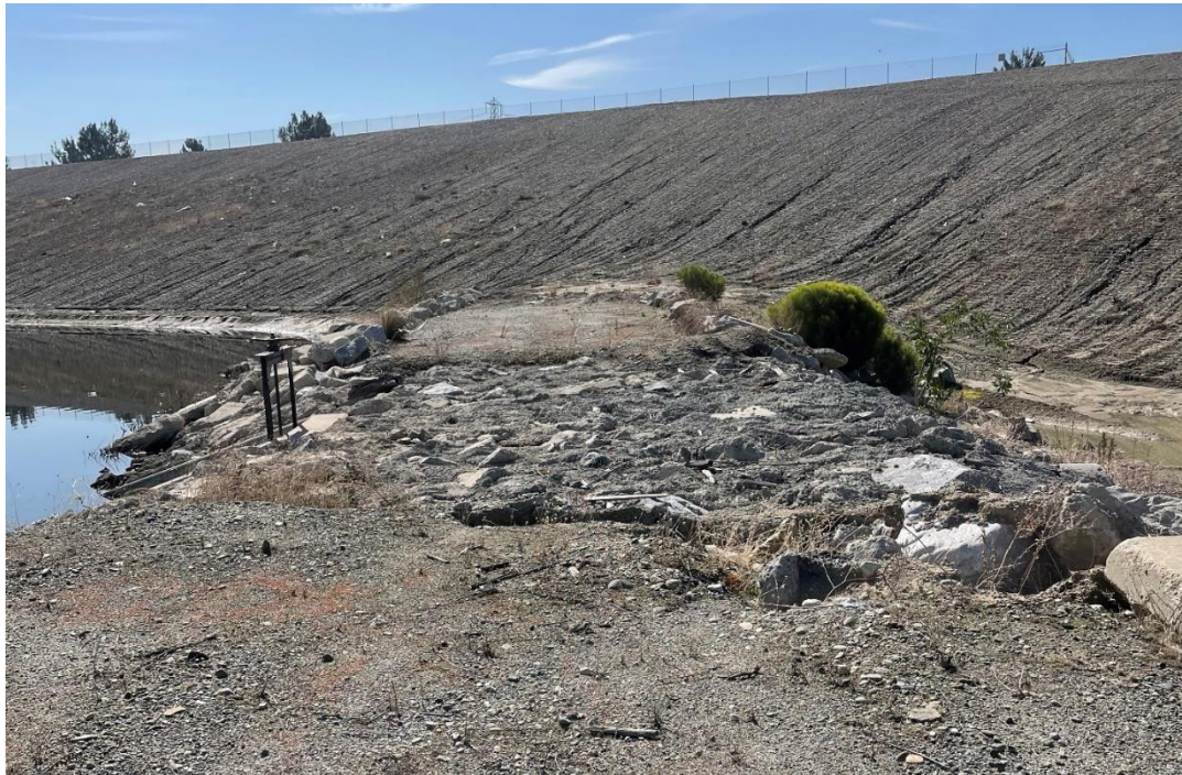
Photo 1 Description Erosion along the Edges of Weir
