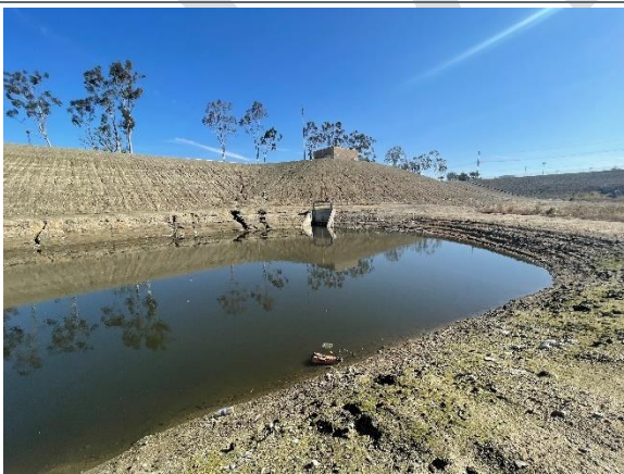
Photo 6 Pump Station Intake Channel
