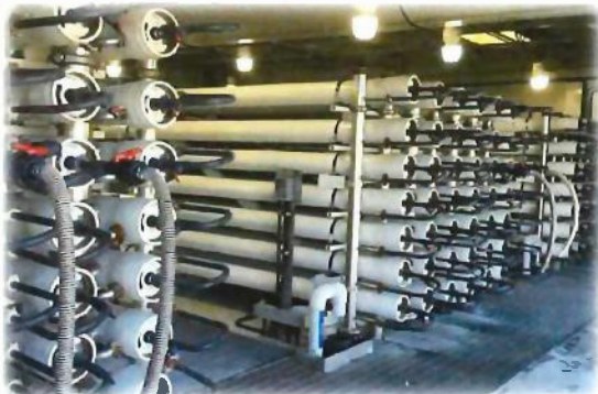
Chino Desalter I Facility
