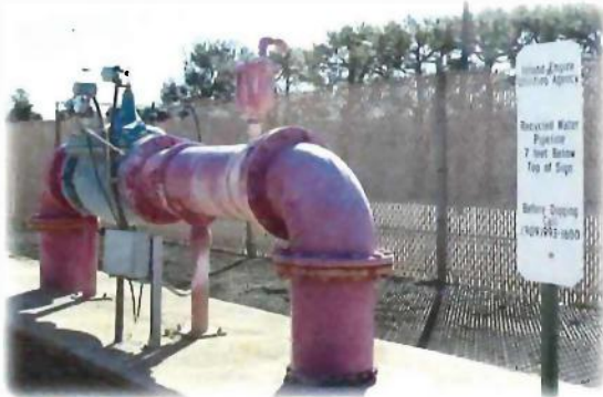
Recycled water line at the Ely Basins.
