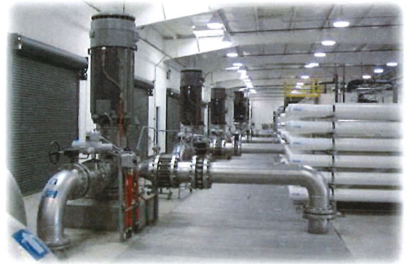
Chino II Desalter Treatment Facility
