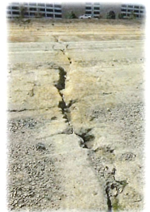
Fissuring at Ely Basin 3
